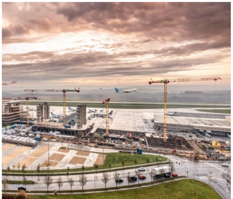
EC-B cranes at work on the construction of the Skypark Business Center in Luxembourg
