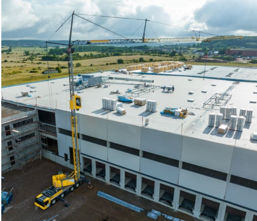
The specialist concept makes the MK cranes mobile and extremely compact. This enables them to achieve a high reach, as demonstrated in Gießen (Germany).
