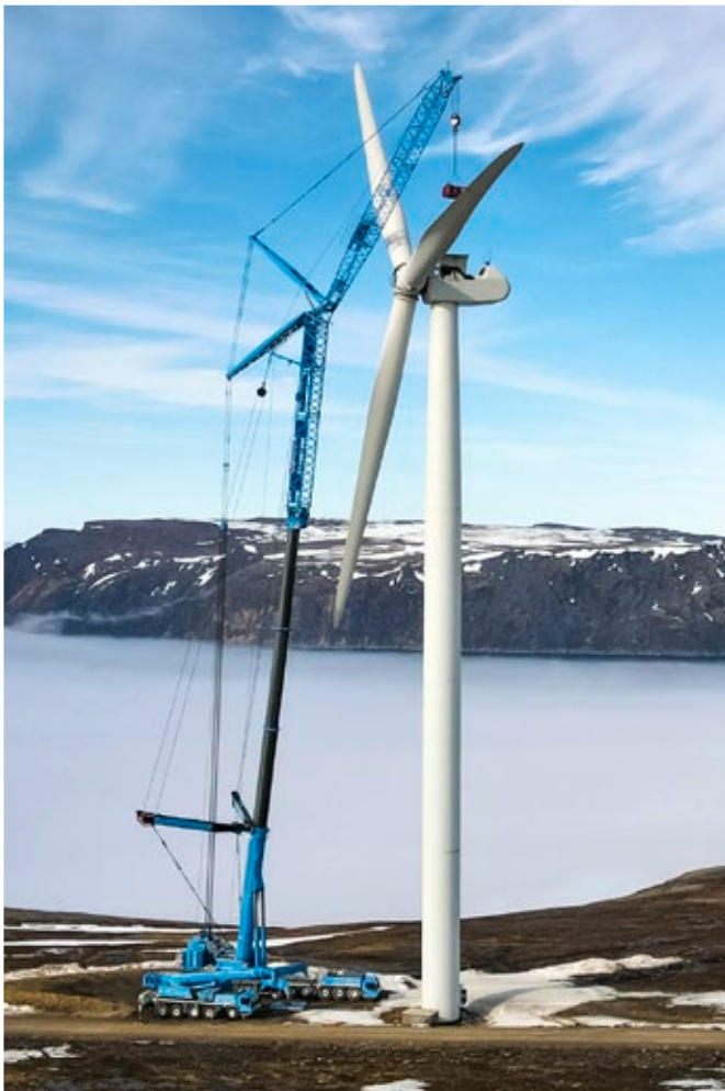
The LTM 1750-9.1 – featuring Y guying, telescopic boom extension and luffing lattice jib – installs a wind turbine in Norway.
