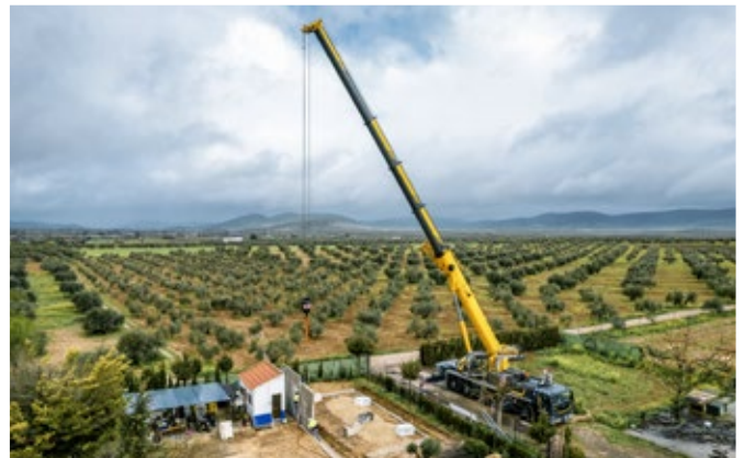
Assembling precast concrete parts in an expansive olive tree plantation – the groundbreaking LICCON3 crane control enters series production with the LTM 1110-5.2.
