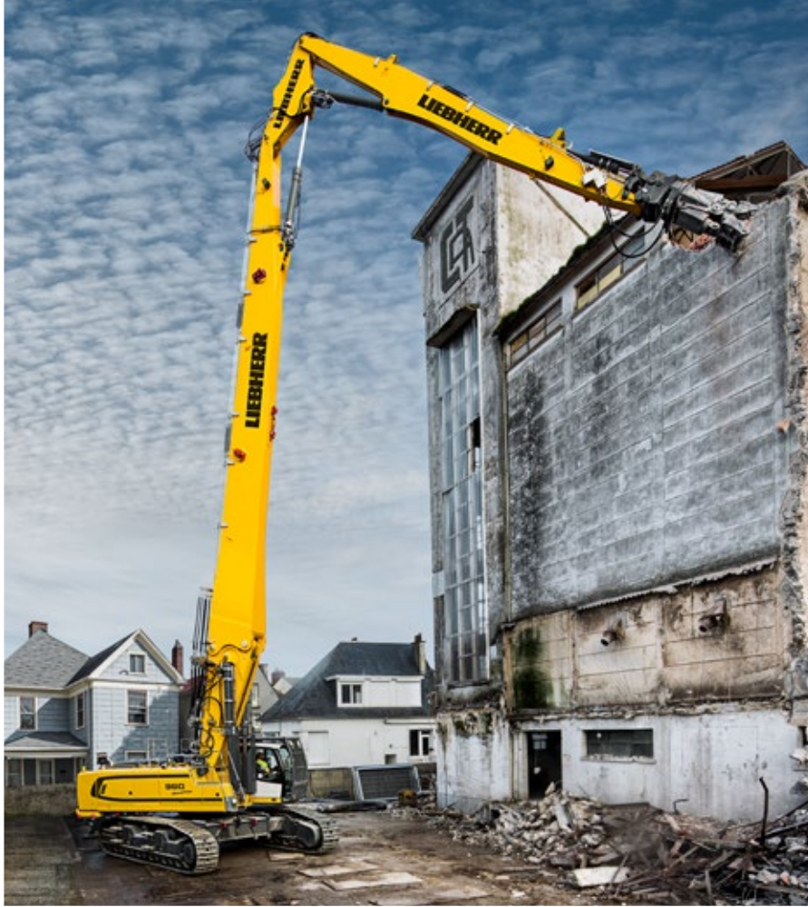
The R 960 crawler excavator used for the demolition of a silo in Frévent (France)
