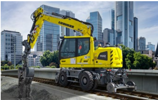
The A 922 Rail in operation for gravel works on a railway line in Frankfurt am Main (Germany)
