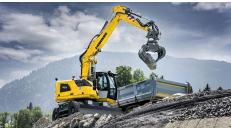
The A 914 Compact Litronic at work on a road construction site in the Oberallgäu (Germany)
