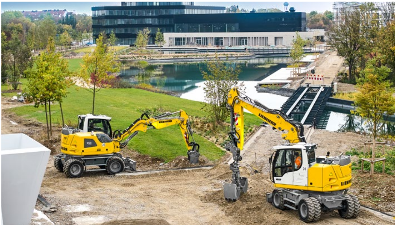
The A 910 Compact Litronic and the A 913 Compact Litronic at work on a landscaping project near Munich (Germany)
