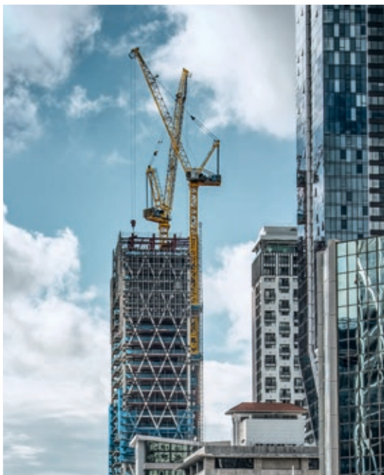
HC-L tower cranes at work on the construction of the Seascape tower block in Auckland (New Zealand)
