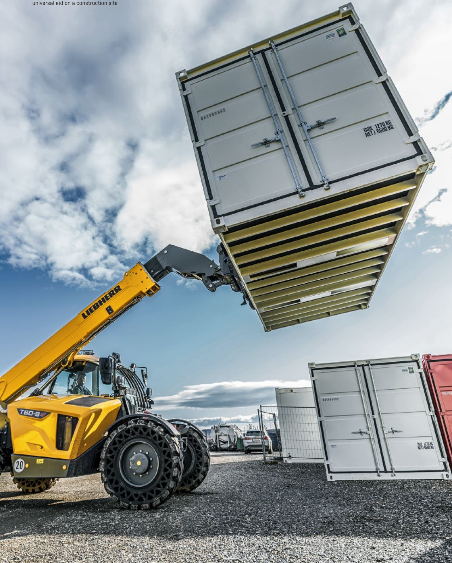
The T 60-9s telescopic handler as a universal aid on a construction site
