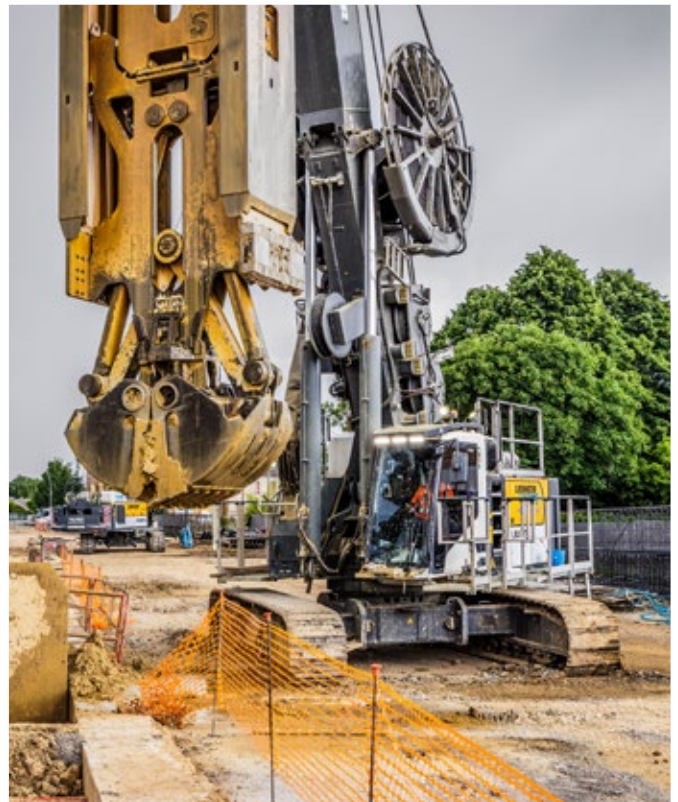
The LBX 600 carrier machine for slurry wall construction in action on a construction site in Forlì (Italy)
