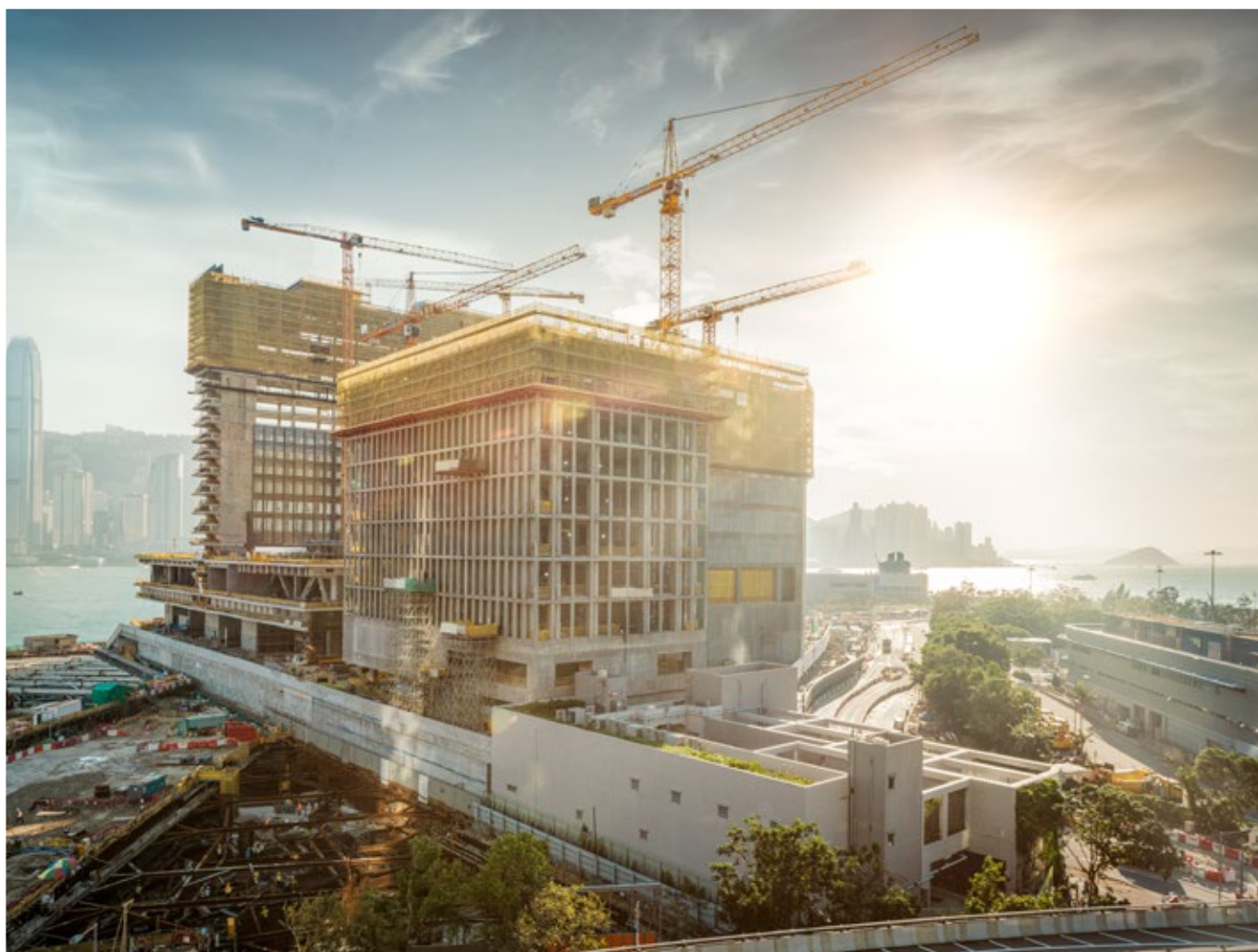
Serving culture and education: top-slewing cranes used in the construction of the M+ museum in Hong Kong (China)
