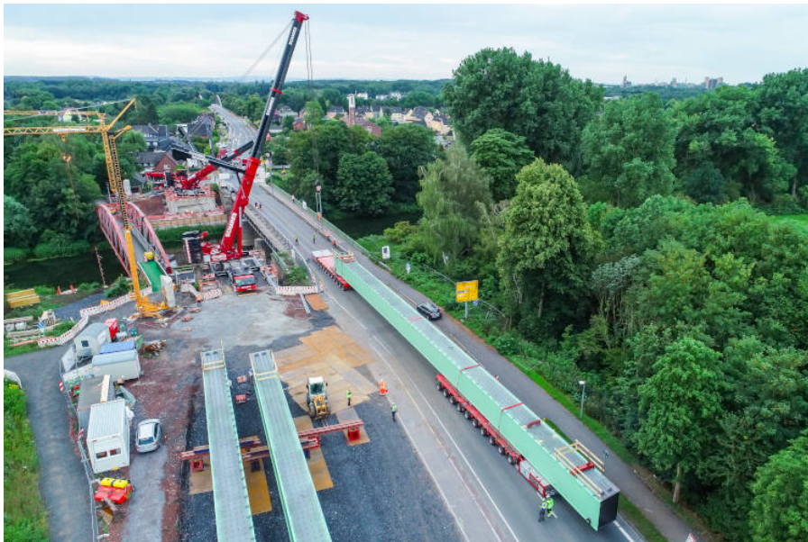
liebherr-schaes-Itm1500-8.1-motive1.jpg SPMTs transport the heavy girders on to the 70 year-old Lippe bridge.
