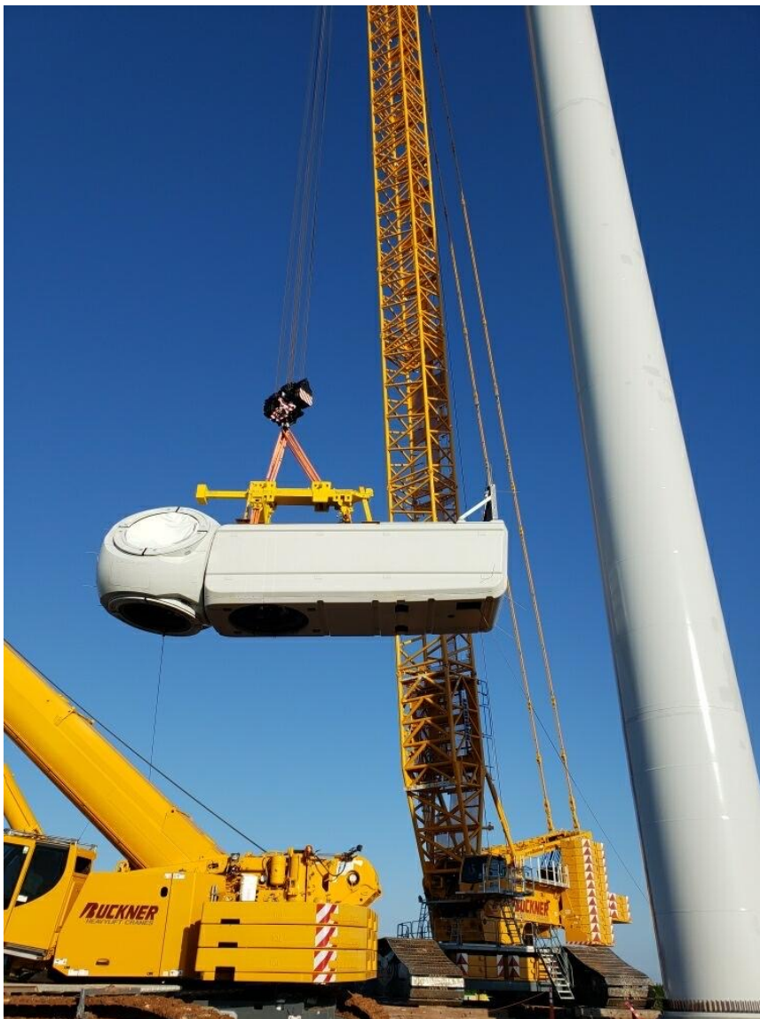
liebherr-lr11000-buckner-sl8f2-motive01.jpg 230 tonne power lift – the complete gondola with the drive system and hub is installed in a single hoist.
