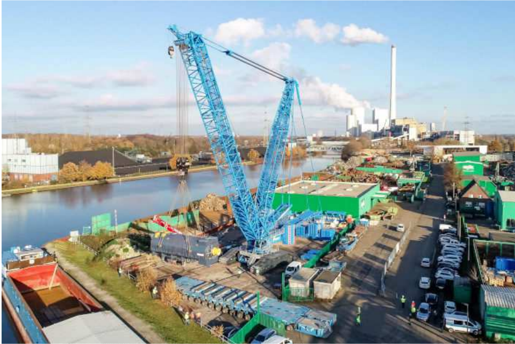
liebherr-felbermayr-lr11000-photo3.jpg The LR 11000 reversed 20 metres with the full load to unload the generator.
