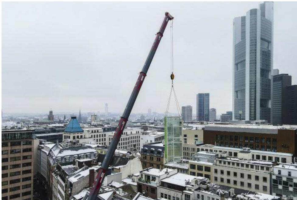
liebherr-ltm1230-5-1-adw-motive02.jpg The components, weighing up to 6.5 tonnes, were installed with a radius of up to 40 metres.
