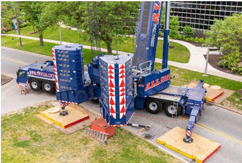
liebherr-all-kran-ltm1650-8.1-ohio2.jpg Set up in a quite tight enclosure, the new mobile crane convinced its owner completely.
