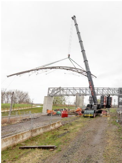
liebherr-all-crane-tandem-hoist-pedestrian-bridge-3.jpg The 450 t LTM 1450-8.1 from ALL placing the left part of the new span.
