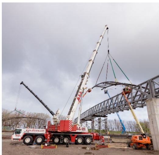
liebherr-all-crane-tandem-hoist-pedestrian-bridge-2.jpg The LTM 1250-6.1 from ALL Crane with the first part of the new bridge span.
