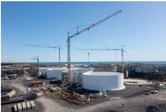
liebherr-island-firstwater-02.jpg Liebherr's reliable and robust crane solutions have supported progress through the first development phases, helping to keep the site on schedule as it works toward full operational capability.
