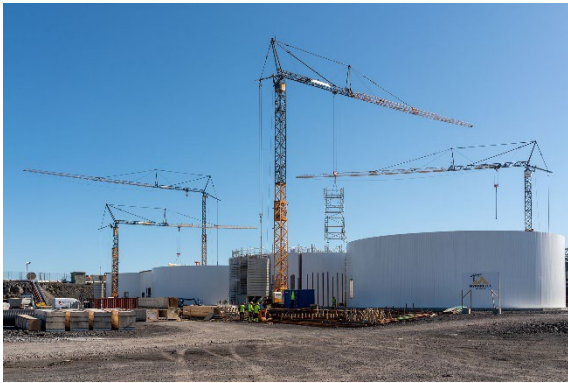
liebherr-island-firstwater-01.jpg First Water's facility is being developed in six phases.
