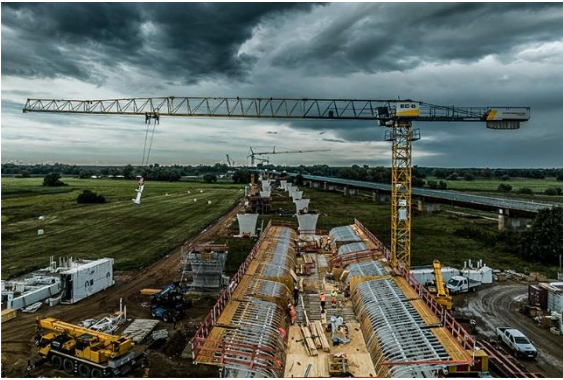
liebherr-125-ec-b-wittenberge-hueffermann-05.jpg First lifts for the new bridge. The parallel running federal highway Bundesstraße 189 can be seen in the background; the existing bridge will remain in place.
