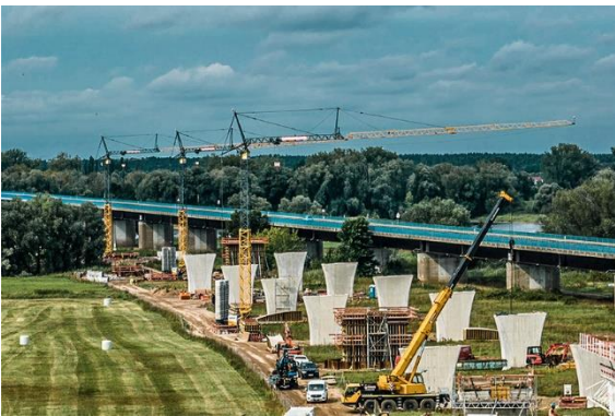
liebherr-125-ec-b-wittenberge-hueffermann-06.jpg As well as the tower crane mounted on the bridge, there are also three Liebherr 81 K.1 fast-erecting cranes on site. Work on the bridge piers is progressing and the first bridge sections are due to be pushed across the Elbe in early 2024.
