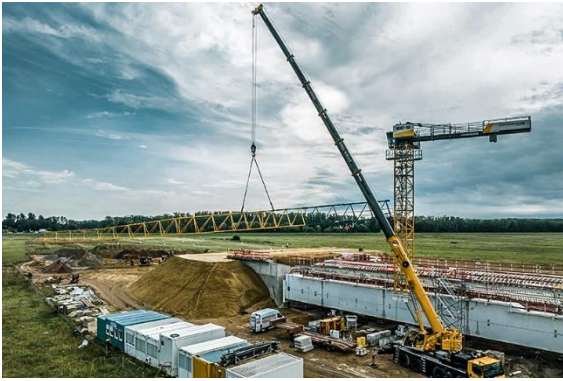
liebherr-125-ec-b-wittenberge-hueffermann-04.jpg Assembly of the 125 EC-B 6 with the help of a Liebherr mobile crane.
