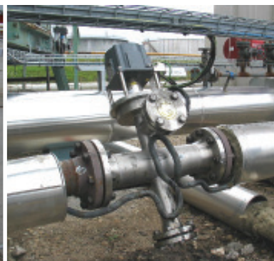
Pipeline installation in an oil refinery
