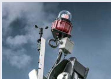
Anemometer & aircraft warning system
