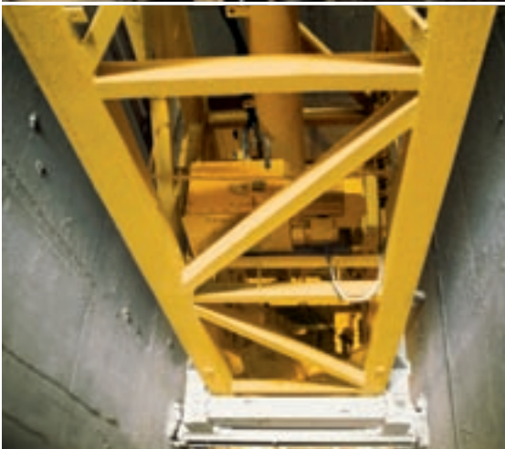
The hydraulic system in the IC tower.
