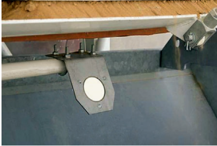
Sensor installed in material chute under silo outlet
