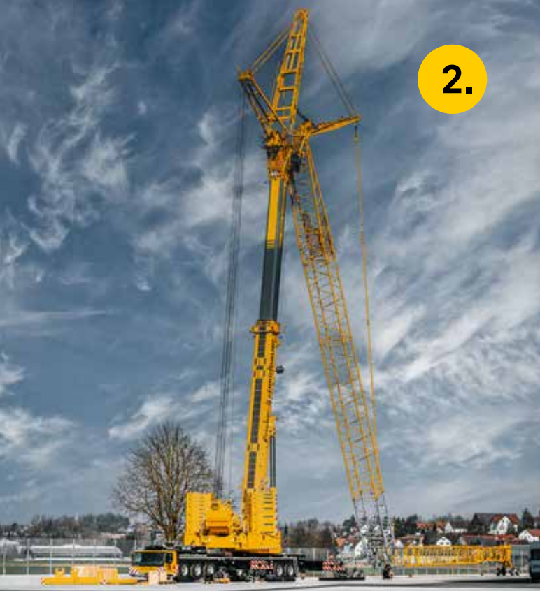
Space-saving The second half of the luffing jib is installed on the first half, which is hanging downwards.
