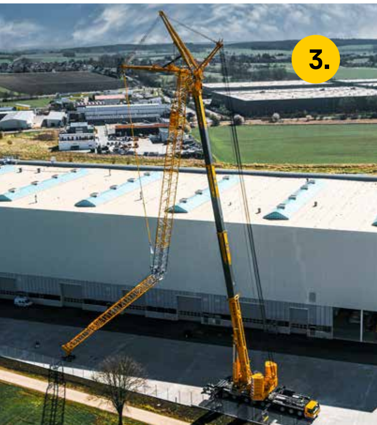
Closing the gap The NK intermediate section is closed by telescoping the boom and raising the luffing jib.
