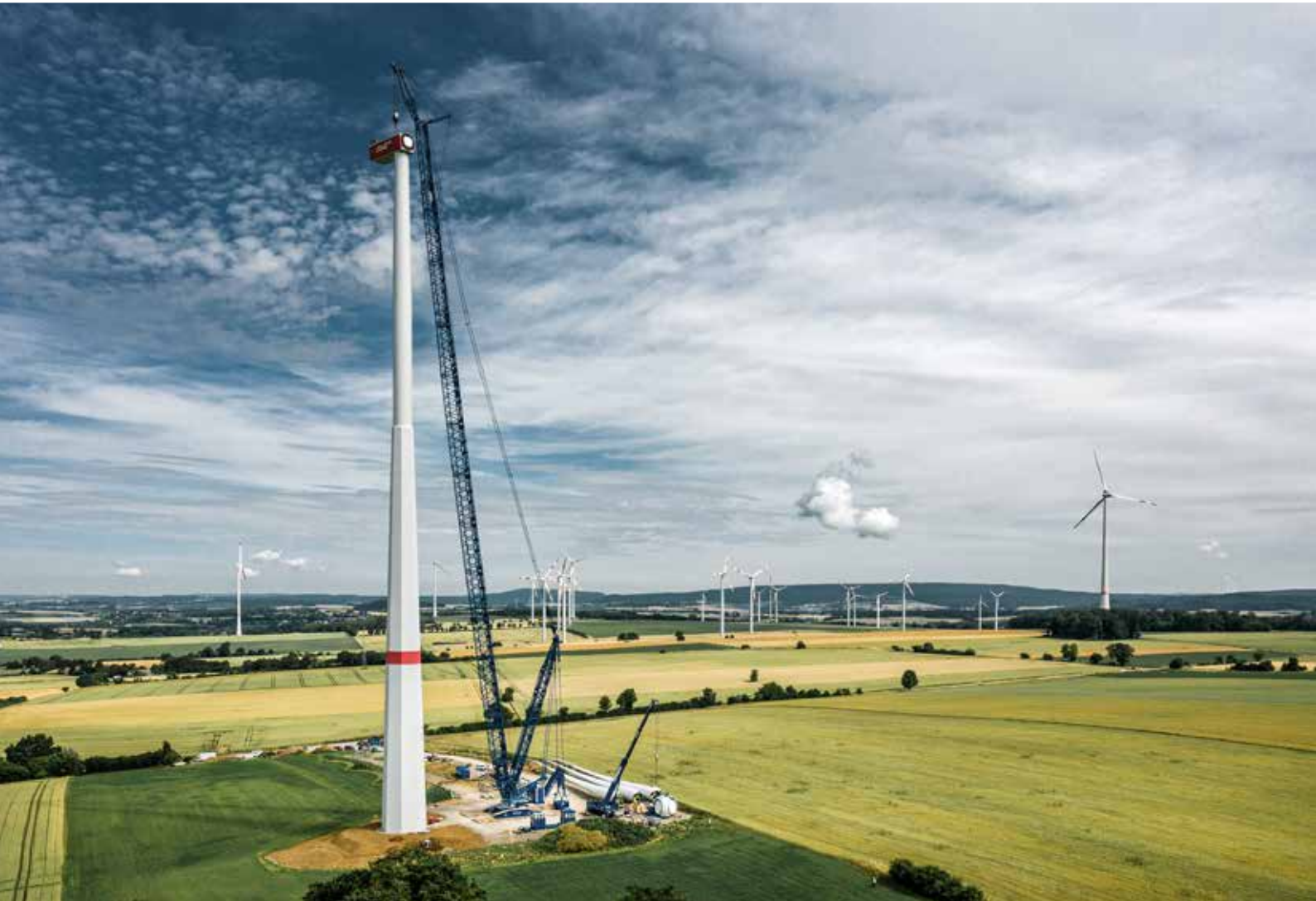
Larger turbines require larger cranes and new technologies. Here, Liebherr is working with customers to develop high-performance technologies for the erection of wind turbines of the future.
