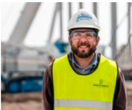
Senior foreman Bruno Valente from Garcia Garcia and crane operator João Neves (above) are in agreement: “An ideal piece of equipment!”
