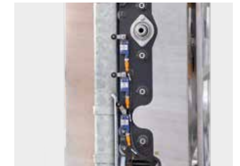
The central limit switch cuts out only in an emergency
