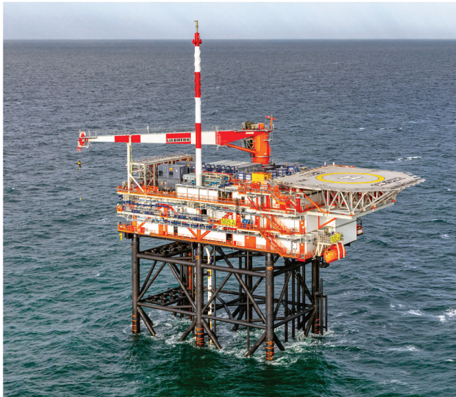
Liebherr offshore crane, type RL 2600, with the fully digital, remote, and semi-automatic maintenance system LiMain at a gas production platform in the North Sea (Germany)
